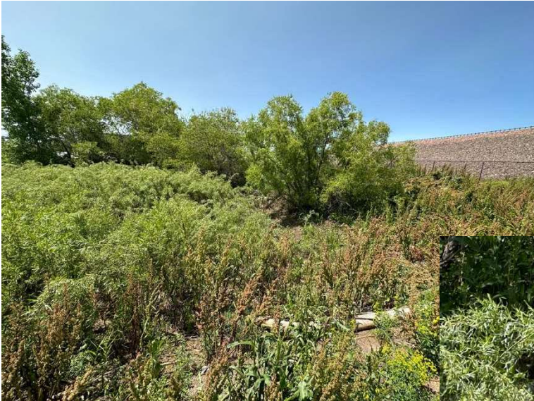
Outlet clogged with plant material
