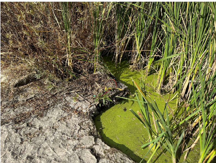
Drop No. 1 outlet structure overtopped and clogged with weeds
