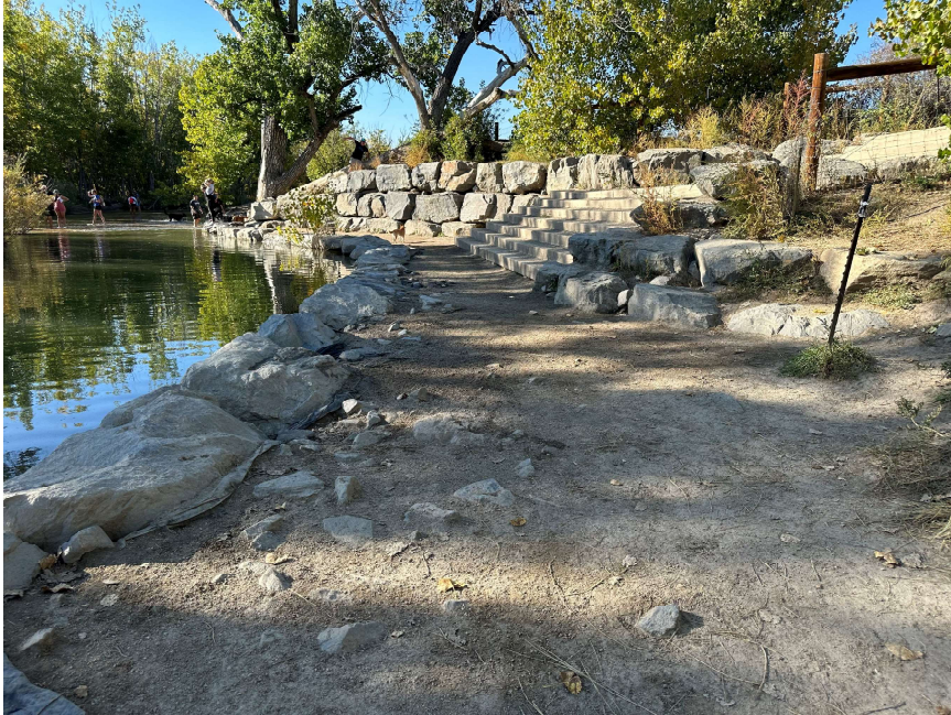
Behind-the-boulder edging erosion at the Fourth Access Point
