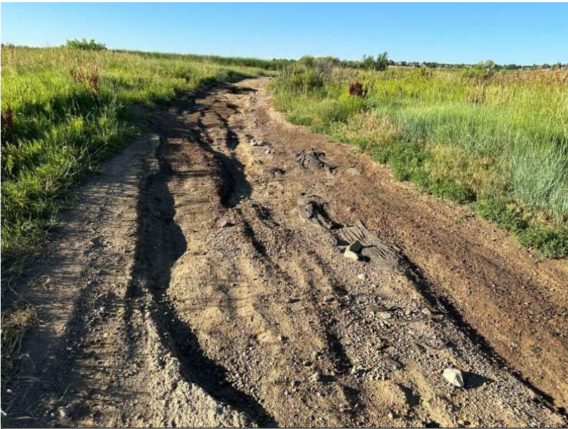
Erosion on access road
