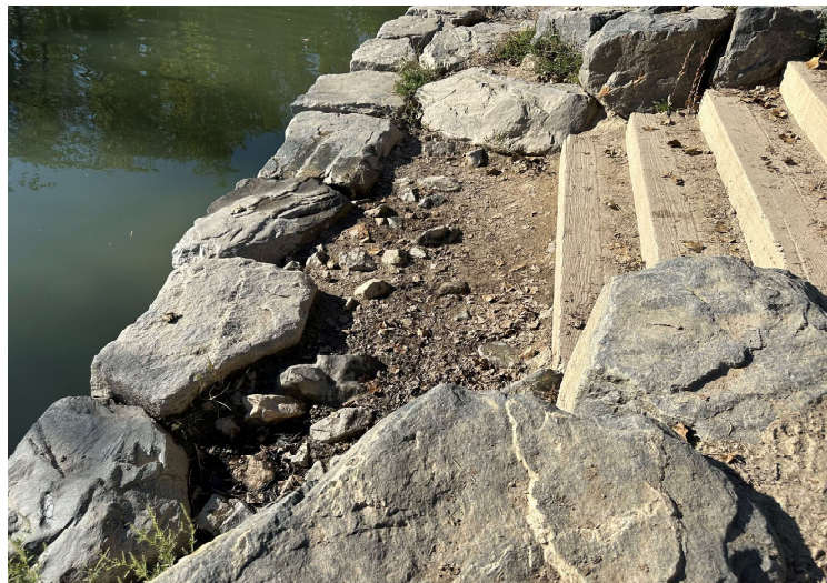
Behind-the-boulder edging erosion at third access point
