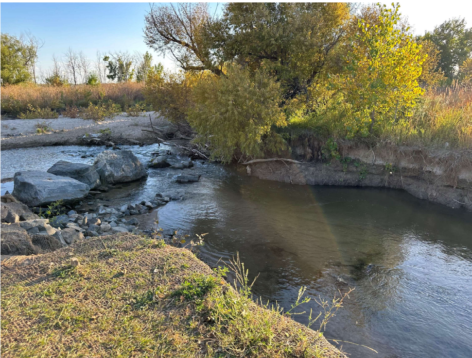
Severe bank and bed erosion downstream of the breakout area
