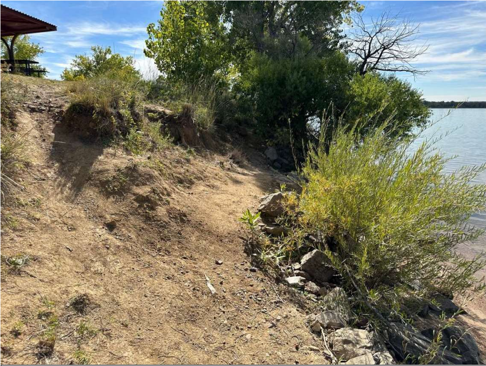
Above flood level bank erosion
