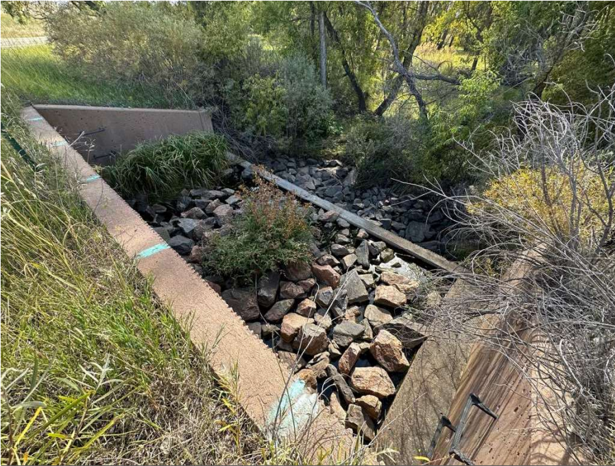
Outlet at Lakeview Dr. becoming clogged with plants
