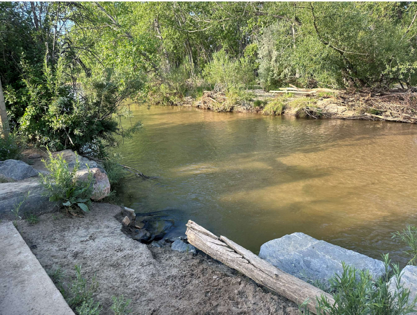
Boulder erosion at Access 6
