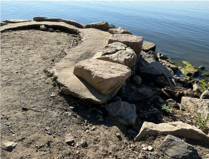
Eroded material from behind the grout at the fishing points
