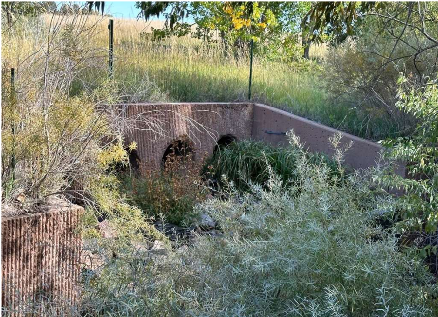
Outlet at Lakeview Dr. becoming clogged with plants.
