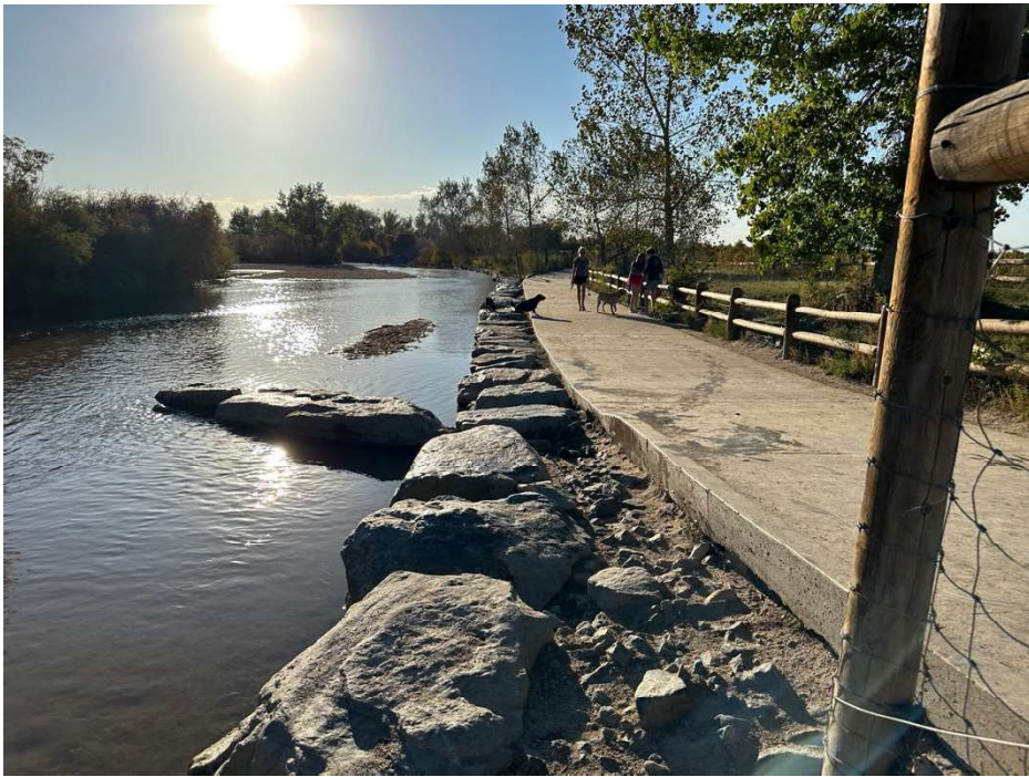
Erosion behind boulders undercutting trail.
