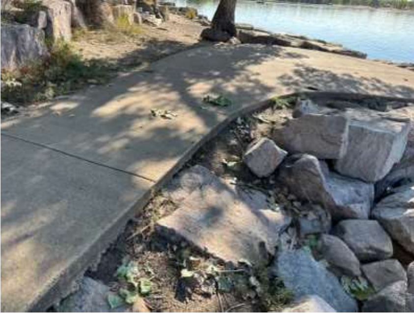
Boulder backfill material washed away from sidewalk
