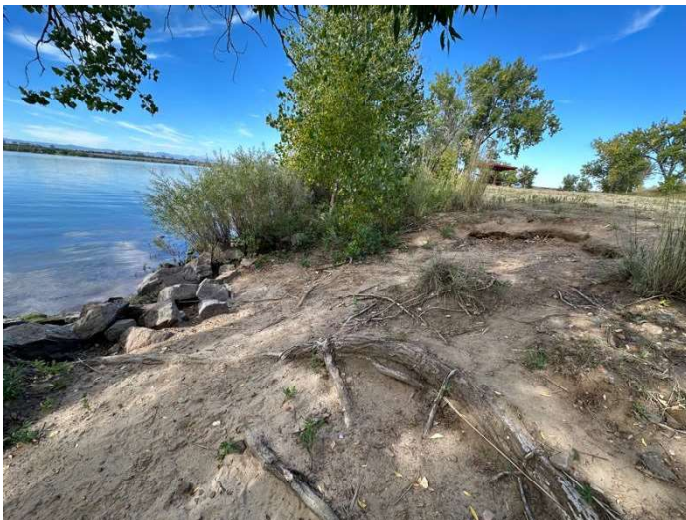
Flood caused above stabilization level erosion
