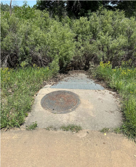
Debris clogging of the outlet structure
