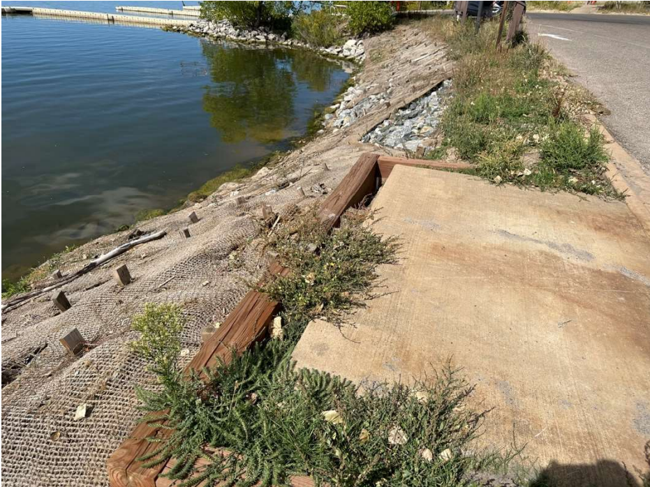
Reseed and mulch 2022 maintenance project, eroded by the floods of 2023-Remove weeds from observation deck.
