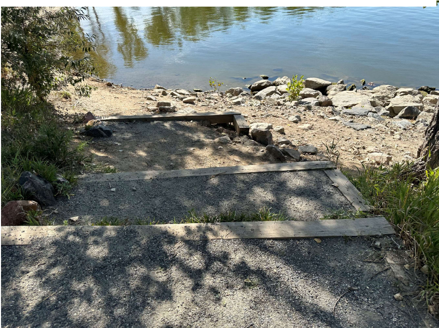
Access steps need CCSP maintenance
