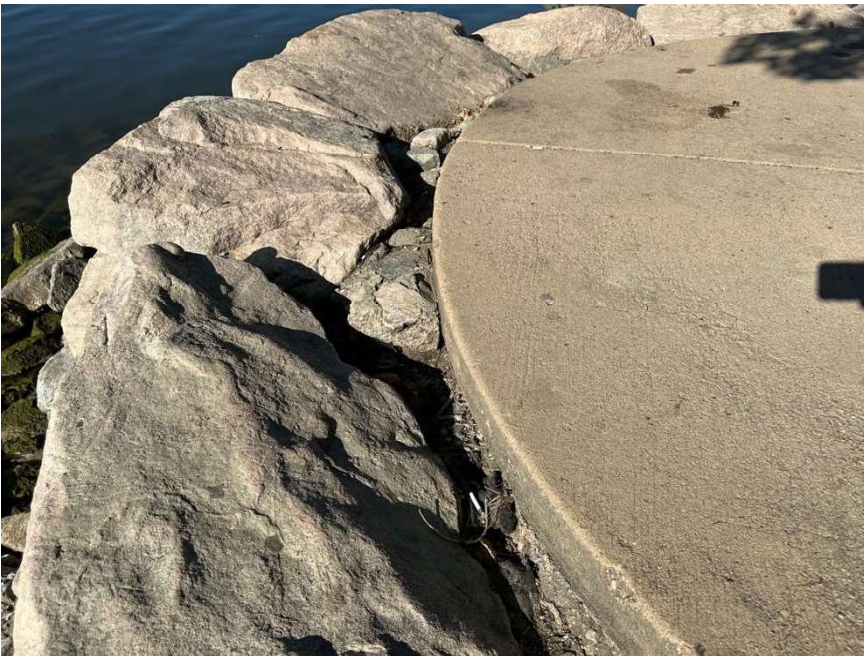
Backfill washed away
