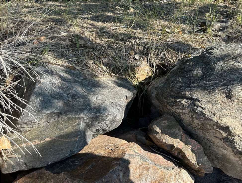
Backfill behind boulders washed away
