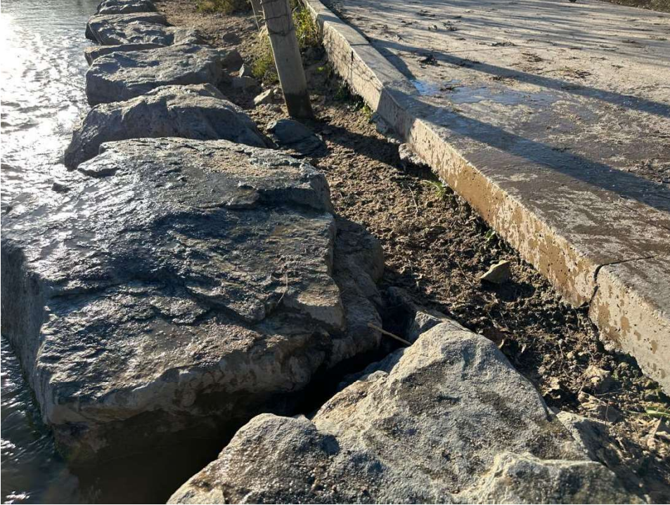
Erosion behind boulders undercutting trail.
