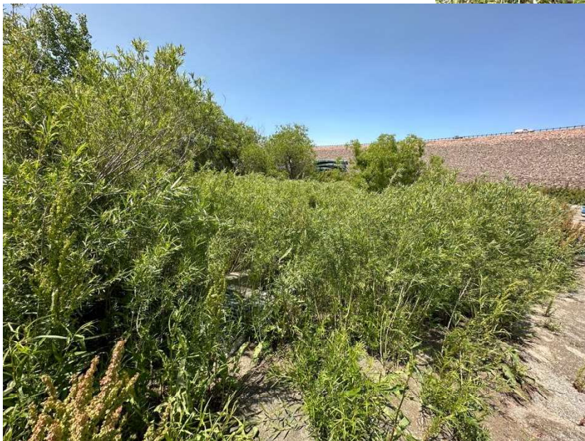
Total facility clogged with plants
