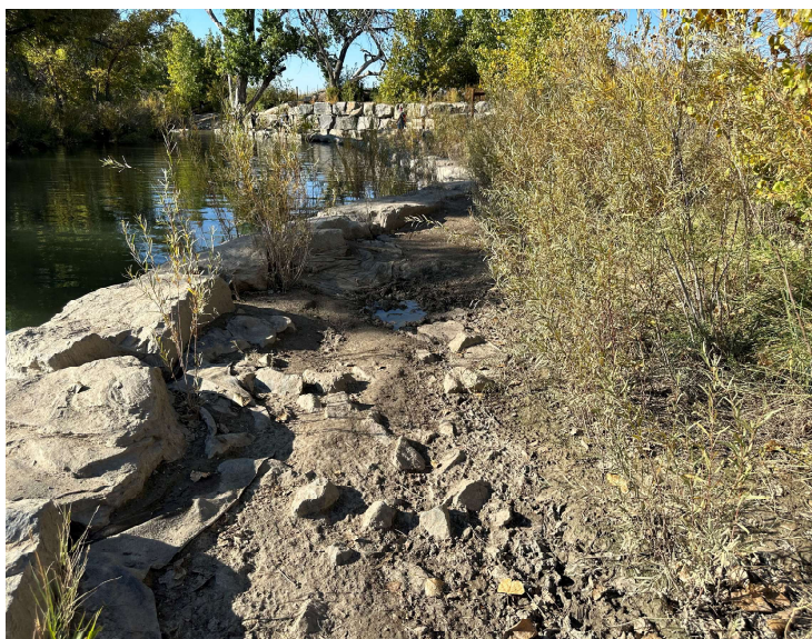
Behind the boulder edging erosion
