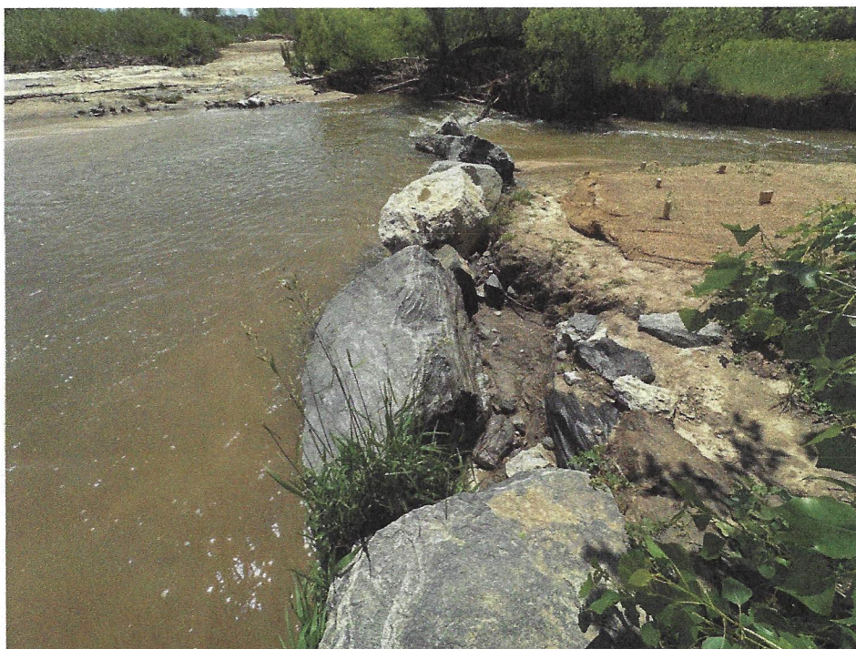
Photo 22-Boulder edging at breakout area severely eroding and disrupting boulder edging,
