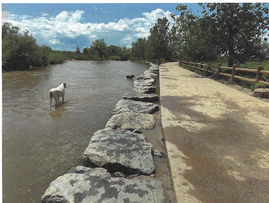
Photo 20-erosion behind boulders and undercutting trail.
