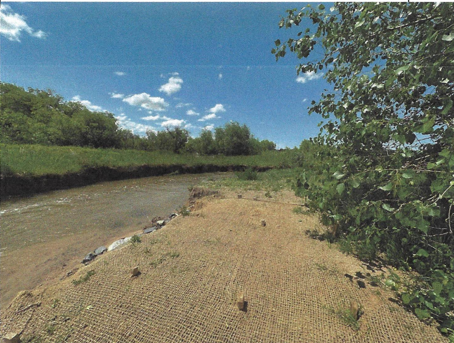
Photo 24-Severe bank erosion downstream of the breakout area
