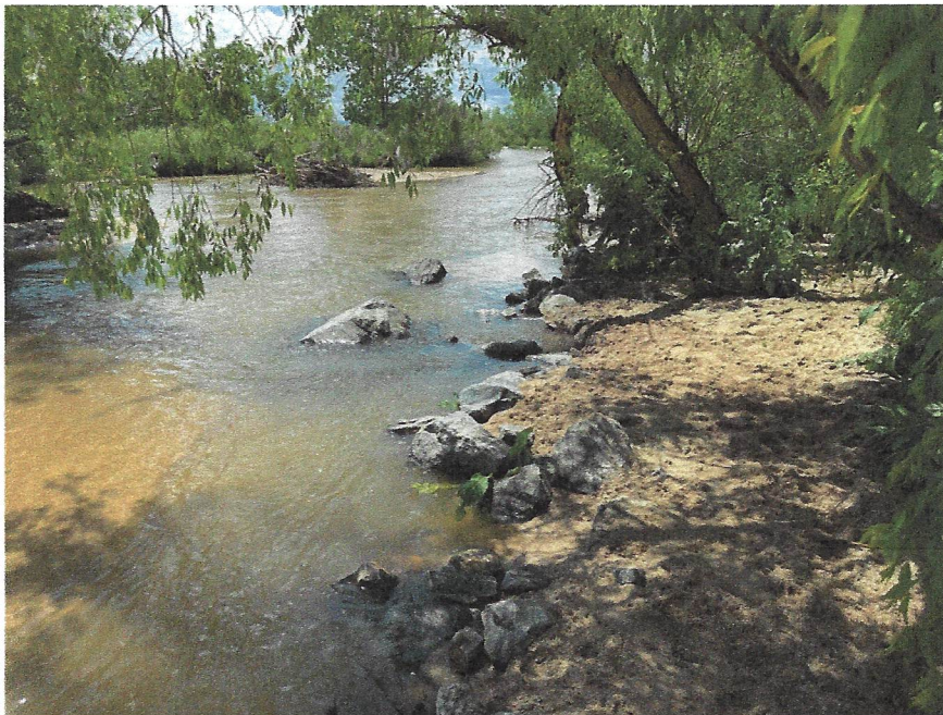
Photo 19- Boulder wall erosion and dislodgment
