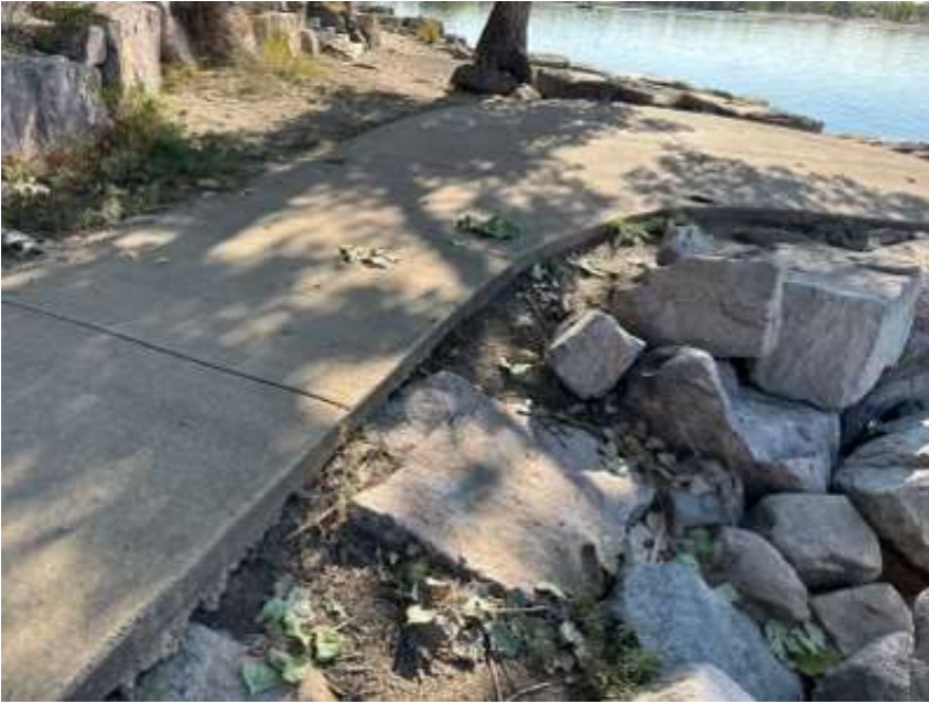
Boulder backfill material washed away from sidewalk
