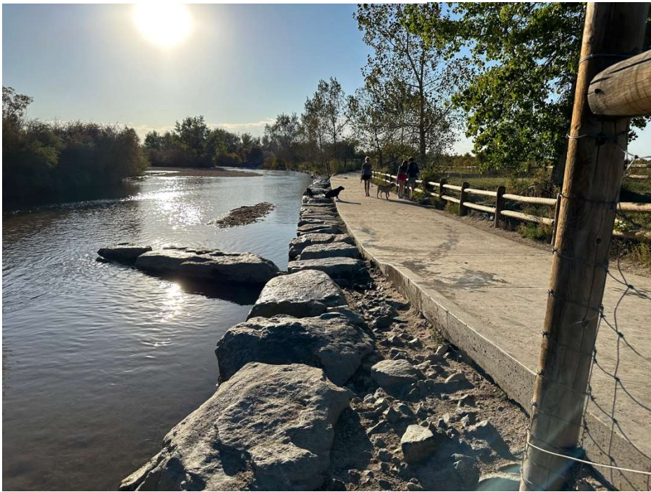
Erosion behind boulders undercutting trail.
