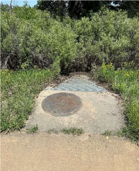
Debris clogging of the outlet structure
