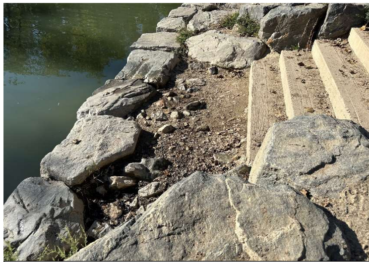
Behind-the-boulder edging erosion at third access point
