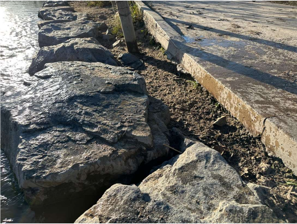
Erosion behind boulders undercutting trail.
