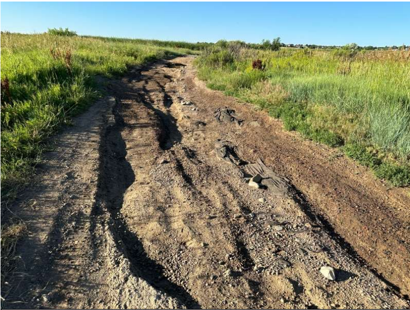
Erosion on access road
