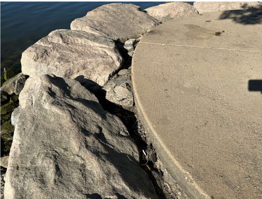
Backfill washed away
