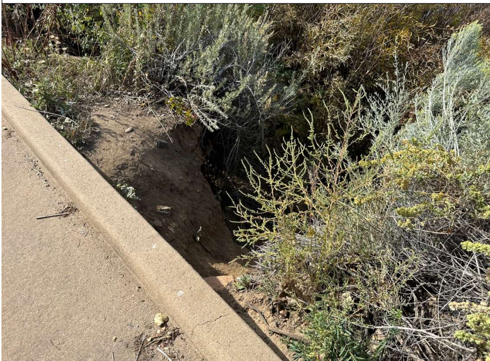
Vertical bank erosion caused by flood overtopping curb and fisherman access.
