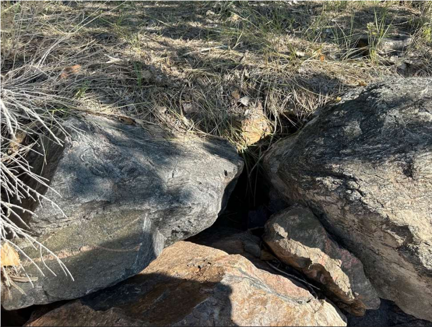
Backfill behind boulders washed away
