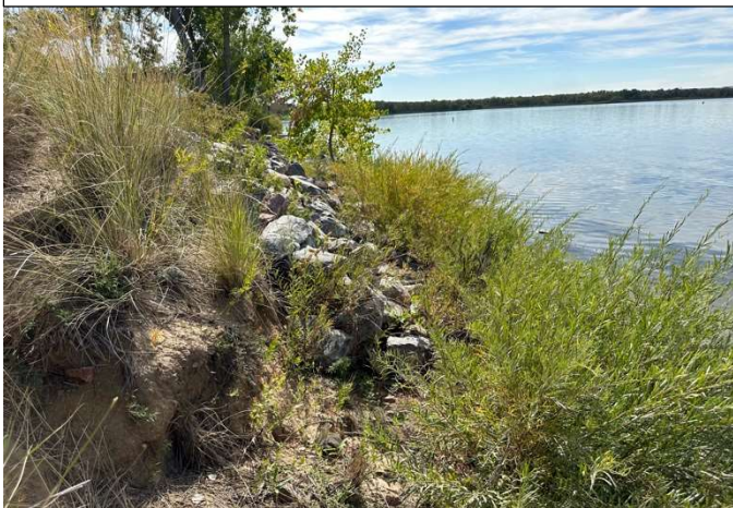
Bank erosion above operating level caused by flood not previously riprapped.
