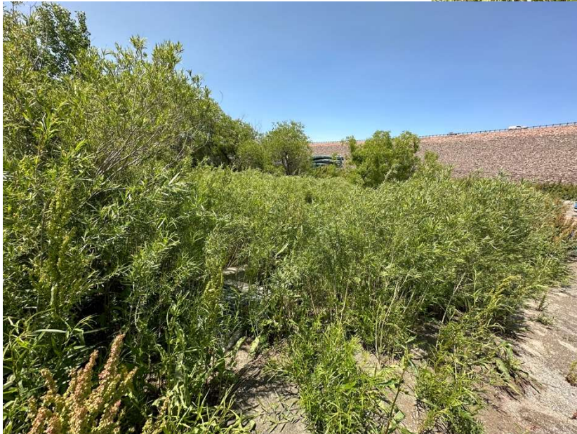
Total facility clogged with plants
