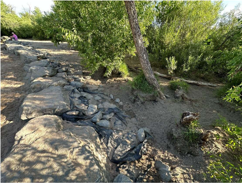
Severe erosion behind boulder edging just before the beach area.
