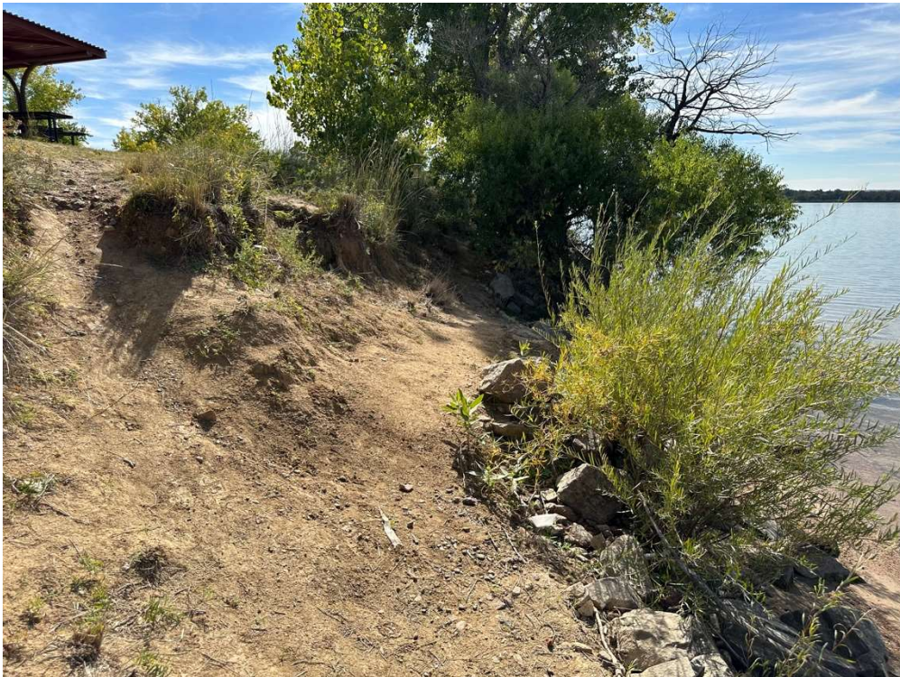
Above flood level bank erosion
