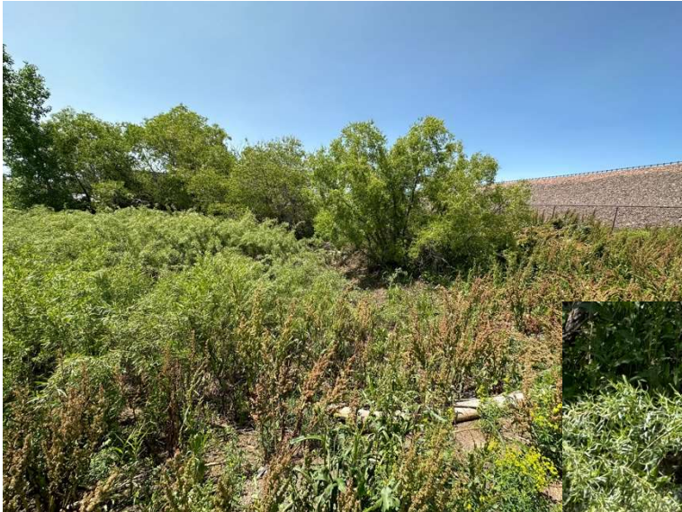
Outlet clogged with plant material
