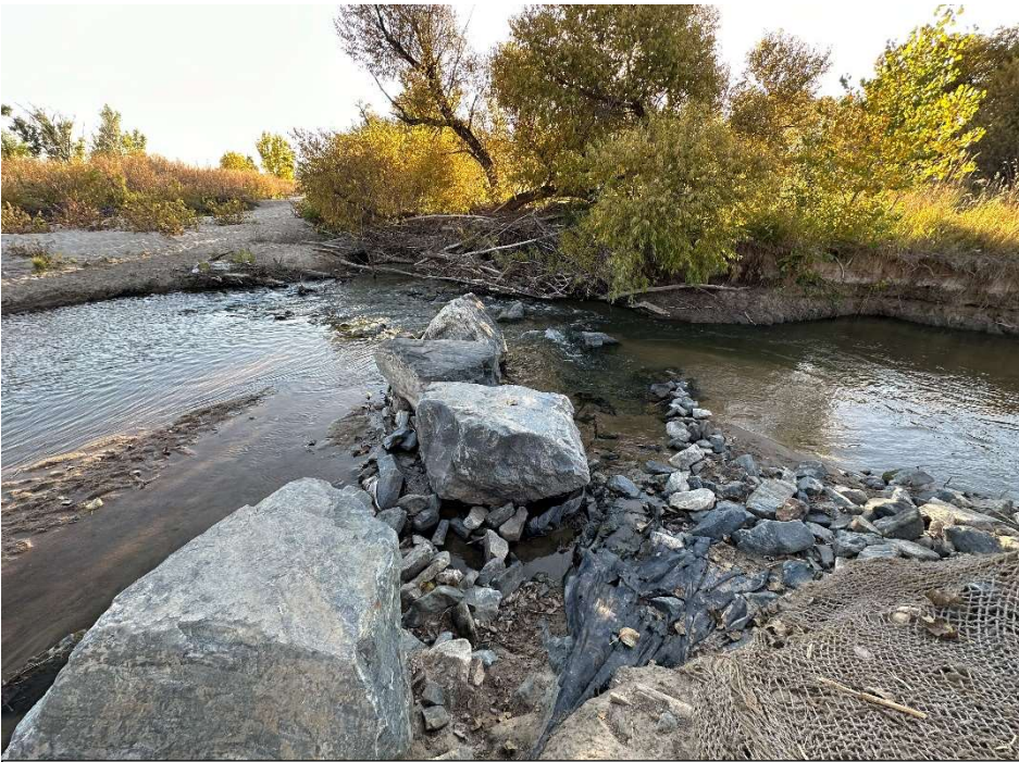
Severe erosion at breakout area
