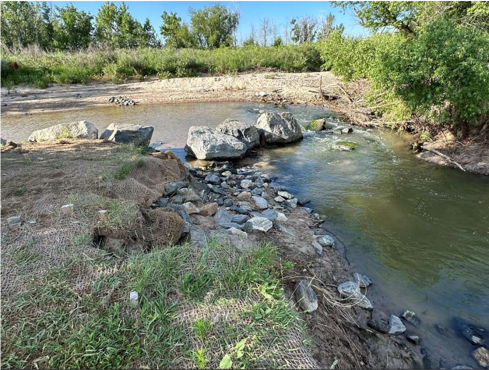
Severe erosion at breakout area
