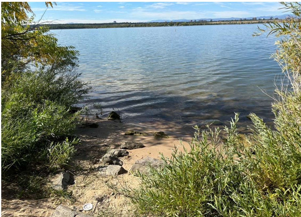
Old riprap displacement judging from moss-laden riprap rocks in the water.
