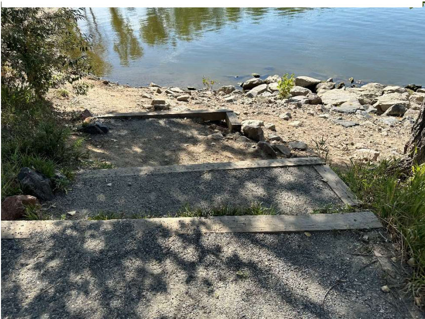
Access steps need CCSP maintenance
