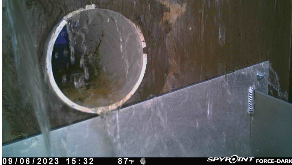
Figure 28. Flow overtopping the outlet box and outflows from the underdrain observed during the first SRT at Smith & Smith
