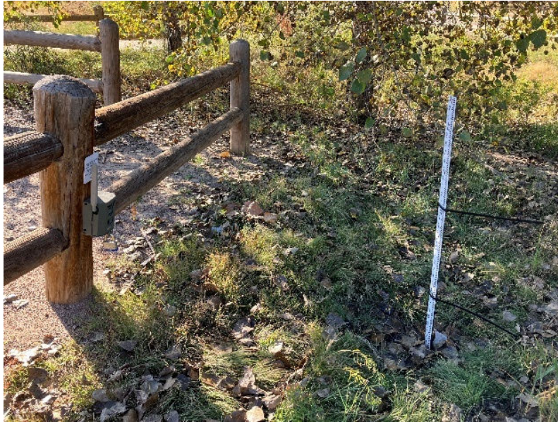
Figure 38. Camera installed adjacent to Mountain Loop swale with staff gauge
