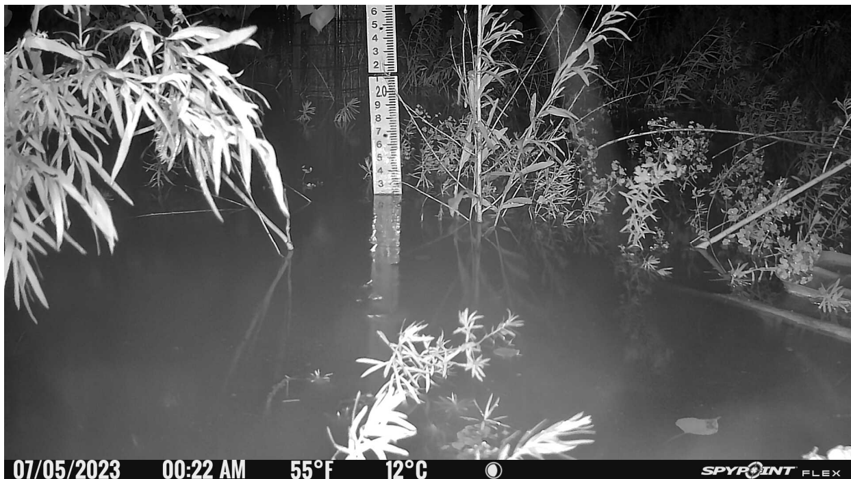
Figure 41. Ponding observed in the Mountain Loop infiltration basin on July 5, 2023
