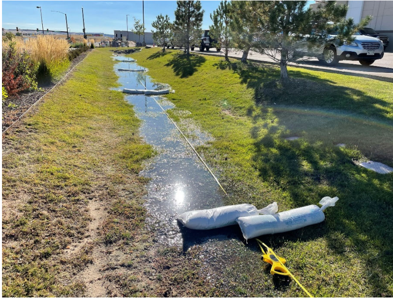
Figure 15. Four sandbag check dams installed at 25, 50, 75, and 100 feet down the length of the grass swale during the fourth SRT at RoadSafe
