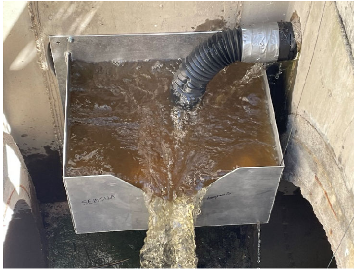
Figure 2. Leaking from the bottom of the underdrain during SRT
