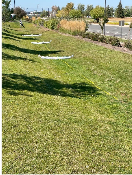
Figure 14. Three sandbag check dams placed at 25, 50, and 75 feet down the length of the grass swale during the third SRT at RoadSafe
