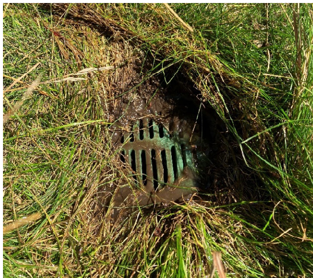
Figure 4. Fourth cleanout discovered during September 6, 2023 SRT
