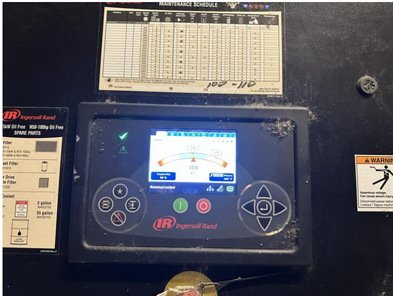
Compressor operating perfectly on a July 19 th checkup
