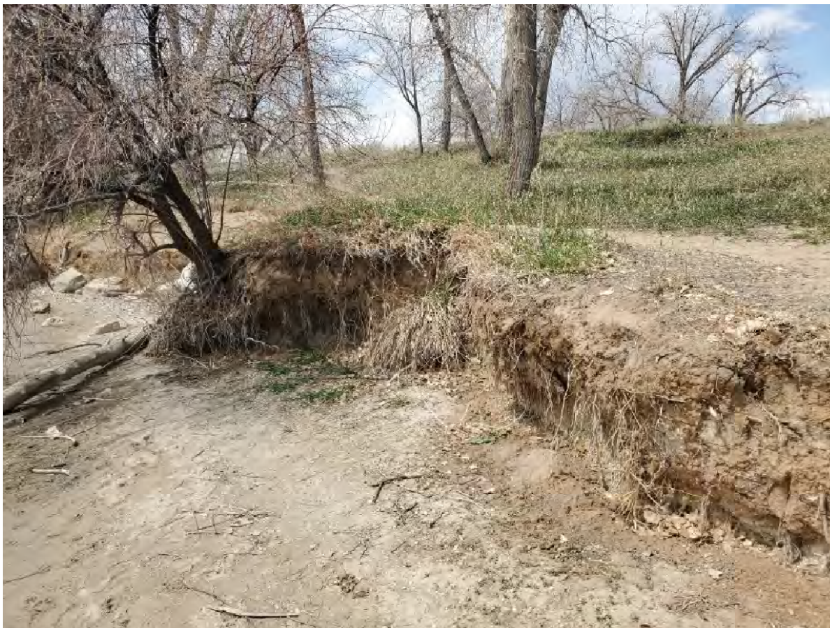
Photo of Tower Loop Shoreline Erosion – Courtesy of RESPEC
