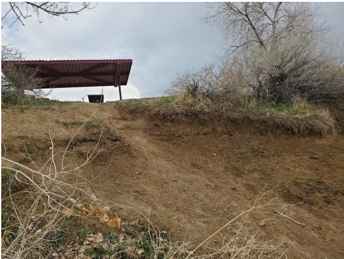
Photo of East Shade Shelters Shoreline Erosion – Courtesy of RESPEC
