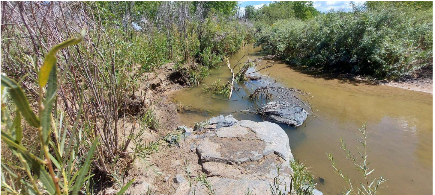
Photo 24 (Bank Erosion at post-storm visit on 8/23/22)
