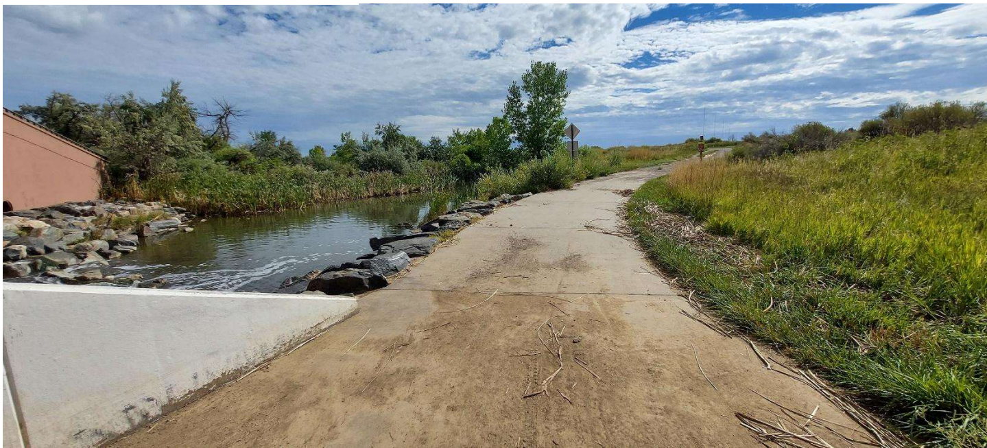
Photo 20 (Post-storm visit on 8/26/22)
