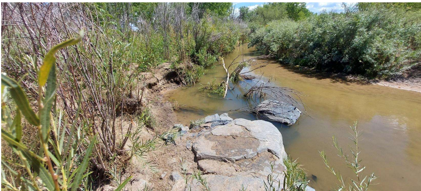
Photo 24 (Bank Erosion at post-storm visit on 8/23/22)
